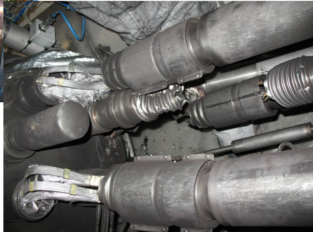
QBQI.27R3 Bellows torn open
